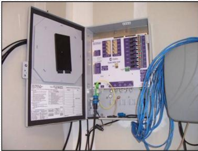
Courtesy Corning Cable Systems
